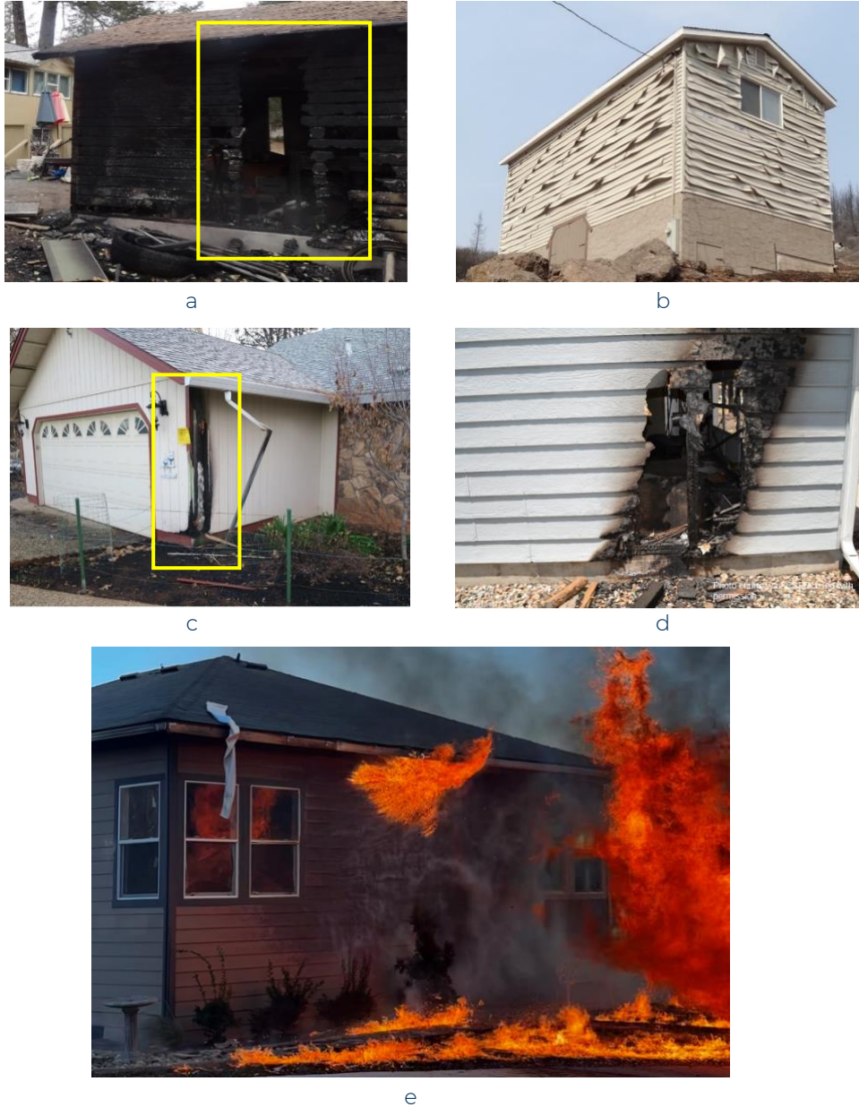
Figure 12. IBHS post-fire investigations show: (a) fire penetration through combustible cladding and vertical flame spread during the Glass Fire (2020) in Napa and Sonoma Counties, California, likely from a burning vehicle; (b) radiant heat damage from surrounding fires (located more than 50 ft away) damaged the vinyl siding, also during the Glass Fire (2020); (c) T1-11 siding ignited due to fire from surrounding vegetation, likely suppressed by first responders during the Camp Fire (2018) in Butte County, California; (d) fire penetration through combustible cladding during the Waldo Canyon Fire (2012) in El Paso County, Colorado ( Maranghides et al., 2015 ); and (e) in the laboratory, the siding of the building ignited during IBHS's full-scale wind-driven building-to-building fire spread tests.
