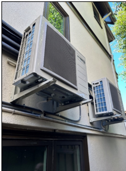
Casa Joaquin Murrieta heat pumps
