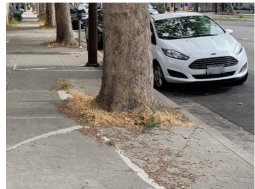
Figure 5.21 Tree on San Pablo Avenue overgrowing a 3 foot by 3 foot tree well
