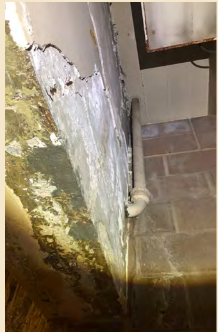
Figure 7.12 Excessive water infiltration at this overhead concrete beam in the basement has caused ferric jacking at the rebar and widespread efflorescence.
