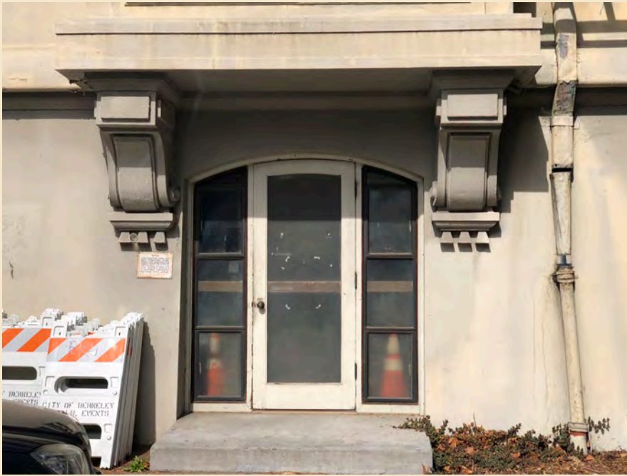
Figure 7.11 At the south entry doors, the original wood side lites have been replaced with inappropriate metal sash.
