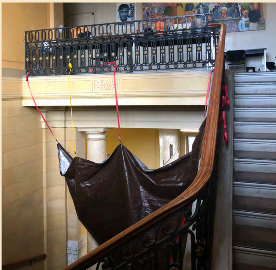
Figure 7.16 The double height space with stairs below at the main staircase will make access to the ceiling and original pendant light fixture difficult.
