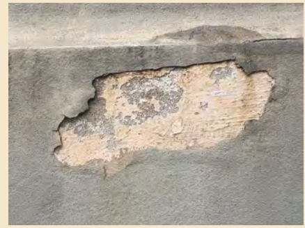
Figure 7.5 At this location on the east elevation, exterior wall coatings have peeled away indicating the many layer of coatings over time.
