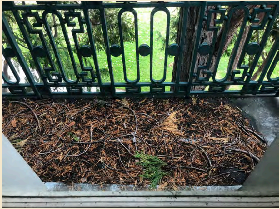
Figure 7.7 Trees in close proximity to the building have caused debris to build up on the balcony floors.
