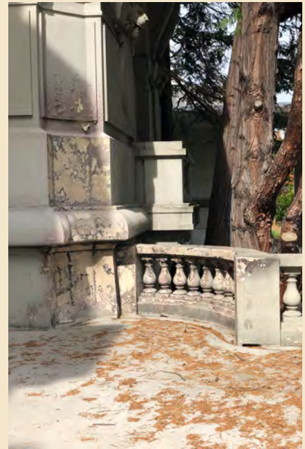
Figure 7.9 A fire started at the north alcove of the entry terrace has damaged the building's exterior finishes.
