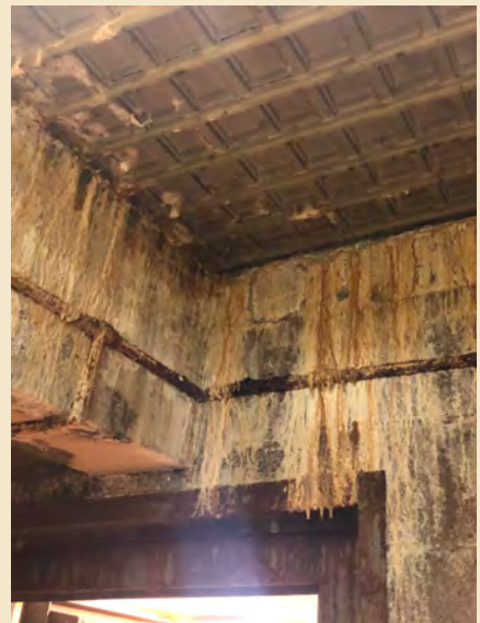
Figure 7.13 The original sidewalk lites of the front entry terrace were poorly infilled with concrete. Salt laden water infiltration has built up over time on the concrete surfaces and electrical conduit below the entry terrace, creating a dangerous condition.
