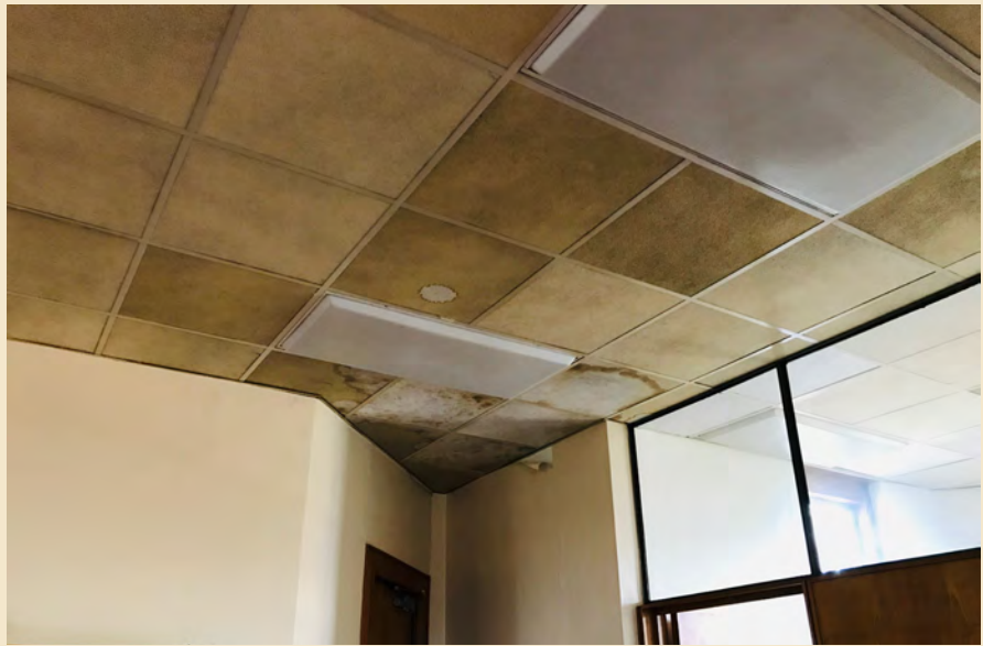
Figure 7.23 The south wing also shows evidence of water damage along much of its north wall.
