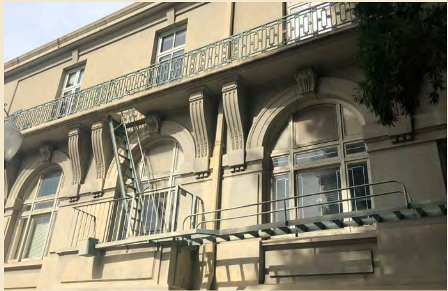
Figure 6.11 First floor balcony and modern metal fire escape at south (side) façade.
