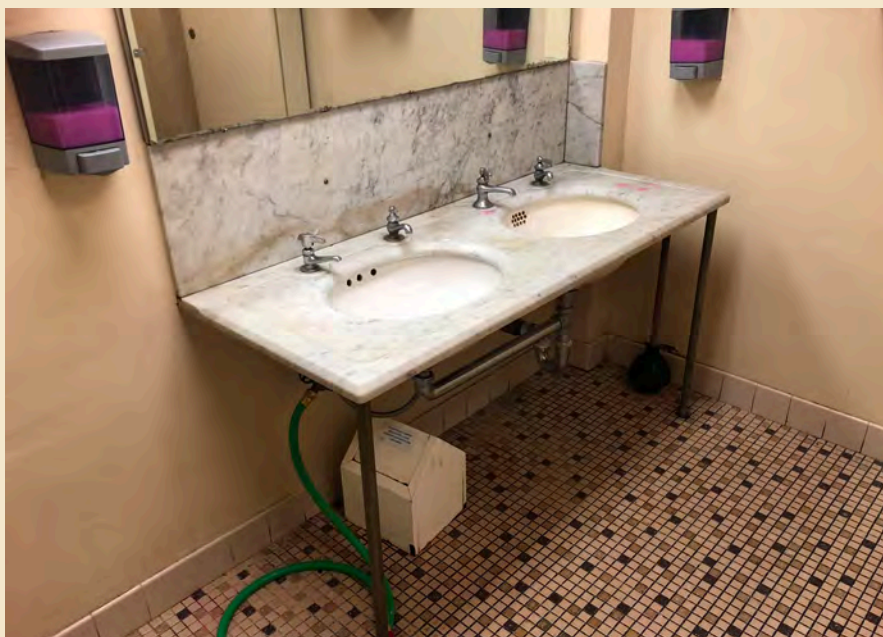
Figure 6.24 Original double marble sink on metal pedestal legs with claw feet located in the first floor Women's Toilet Room.
