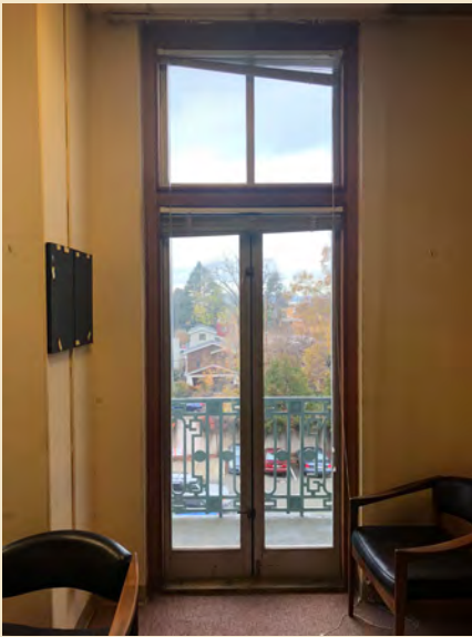
Figure 7.8 At the second floor south wing, the double hung wood windows have been replaced with inappropriate aluminum casement windows.
