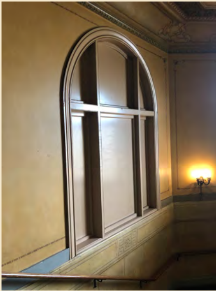
Figure 7.17 The additions to the north and south of the stair tower caused the original windows to be infilled, changing the character of the space.
