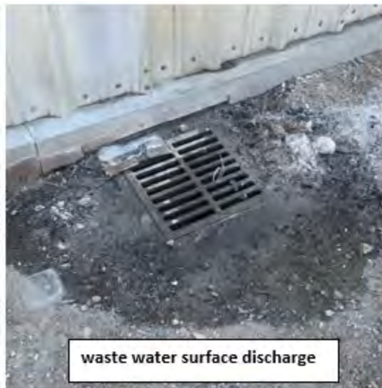
Imminent Health Hazard - Storm Drain
