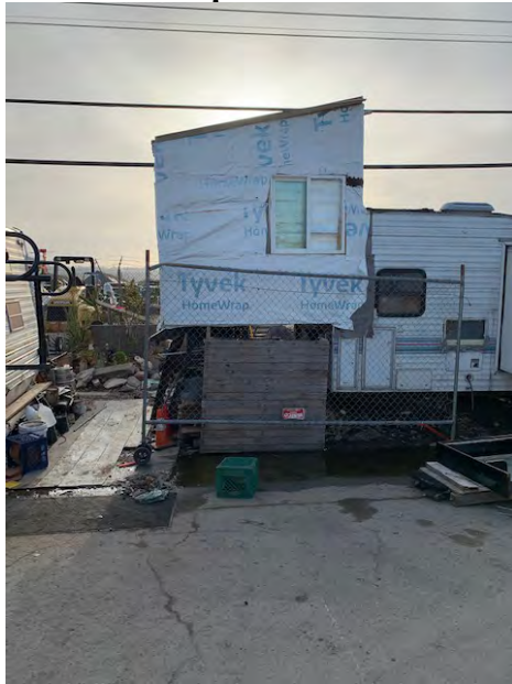
2 nd and Jones (Unsafe Structure)- Before
