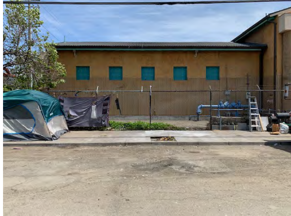
2 nd and Page (Unsafe Structure)- After
