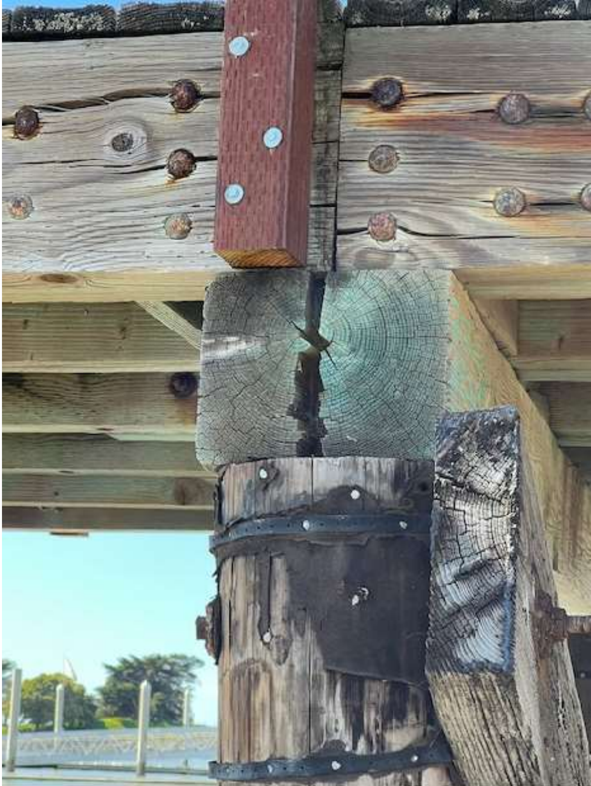
East dock, 3-6-2025, 12:03 pm, about zero tide, looking at end of transverse beam, note crack
