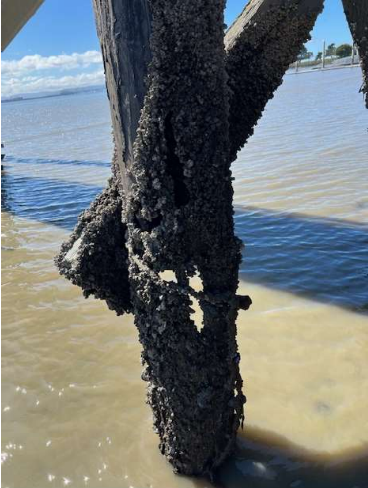
East dock, 3-6-2025, 11:32 am, about zero tide, note upwards extent of crack
