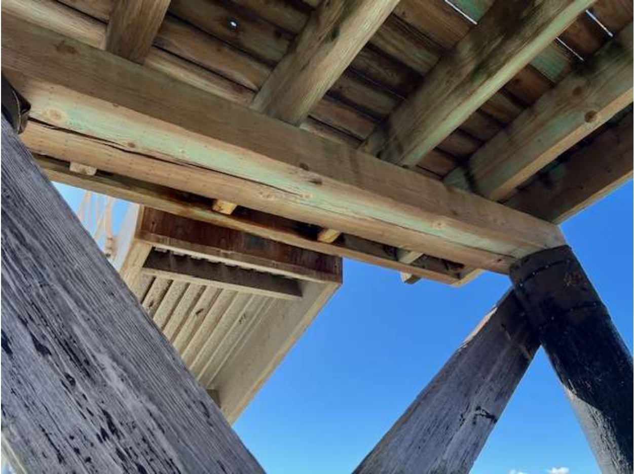
East dock, 3-6-2025, 11:32 am, about zero tide, looking up at transverse beam, note crack
