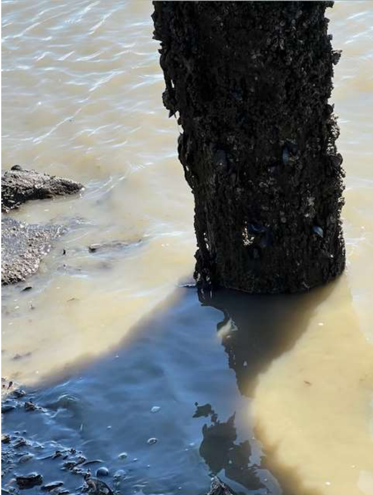
East dock, 3-6-2025, 11:31 am, about zero tide, note lower extent of crack
