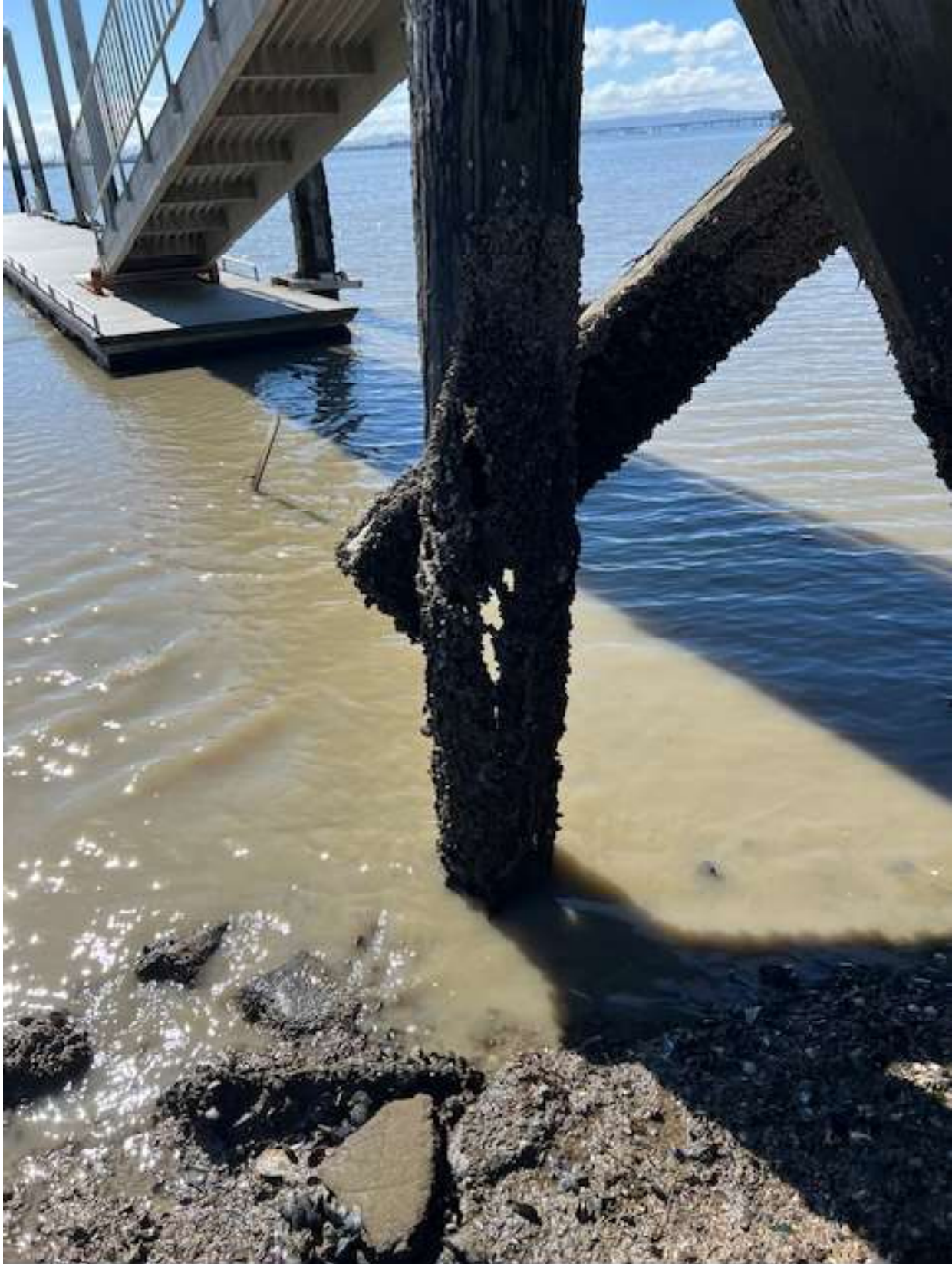
East dock, 3-6-2025, 11:31 am, about zero tide, note thru crack, piling hollowed out
