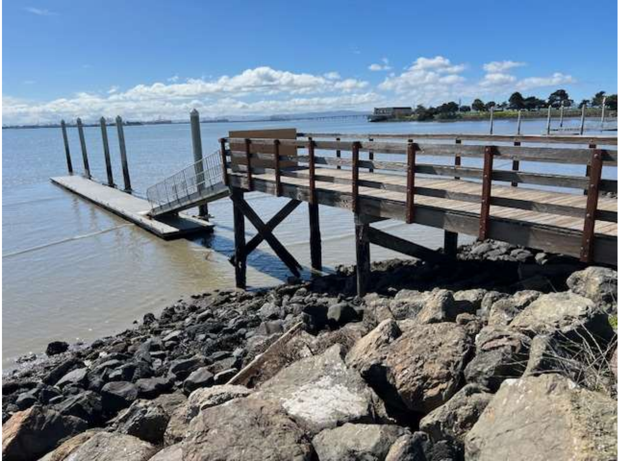
East dock, 3-6-2025, 11:28 am, about zero tide. Note diagonals out of place.
