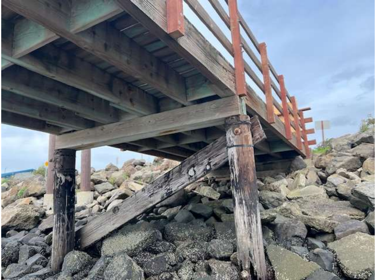
Onshore pilings into riprap also distressed at bottom end
